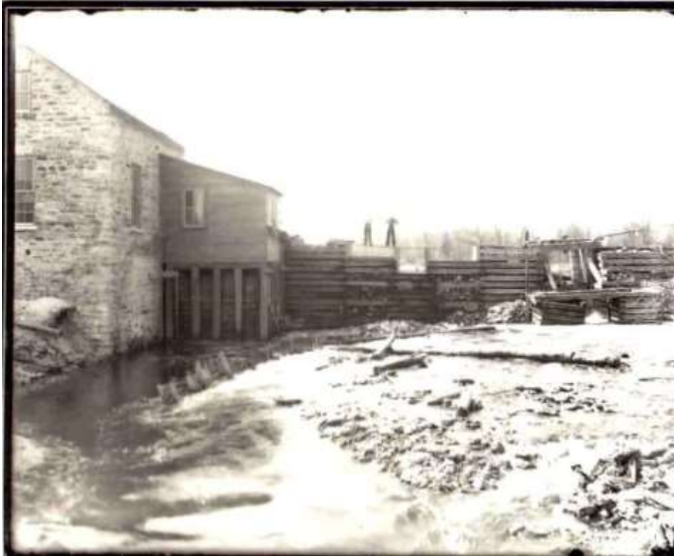
The Bowes Mill dam under re-construction, date not known; possibly taken following a fire or being converted for Perth Power (Photo – Perth Museum)
